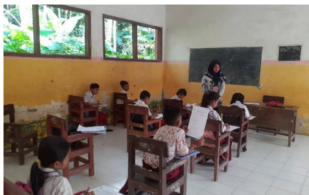
Fig. 2 Mossy classroom walls and peeling paint
